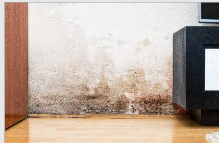
Damp wall without application of Nitoproof Damp Protect
